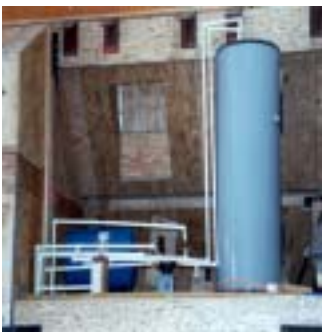
Expansion tank that holds pressure in the water lines running from the hot water tank.
