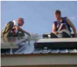
Matt Edmondson and Brian Mcgee inspect the Fast Jack system so the Photovoltaic panels can be properly installed.
