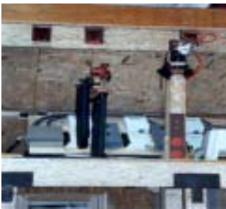
View of heat exchanger used in the hot water system to transfer heat from Glycol to water.
